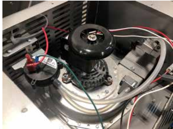
Pressure switch installed
