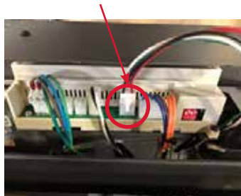
New Wiring Harness
